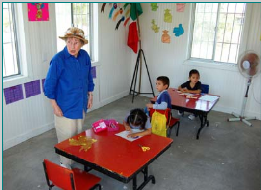
New classroom replaces old unsafe one (see ceiling damage) at Obregon School.
